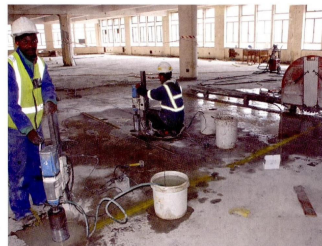
Core drilling and floor sawing using Diamond Products tools to cut through the floors of one of the buildings as part of the refurbishment programme.
