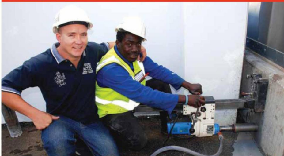
Purple Moss managing director, Martin Marks (left) and Blessing Bere, concrete core drilling.
